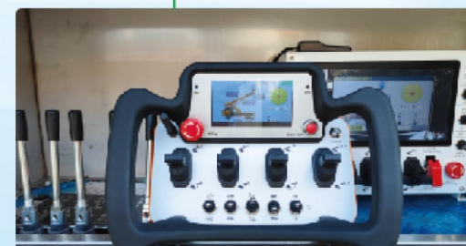
09 Electric control operation system
